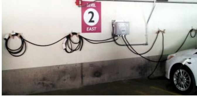
Figure 3. Realization of 4 channel smart charging box
